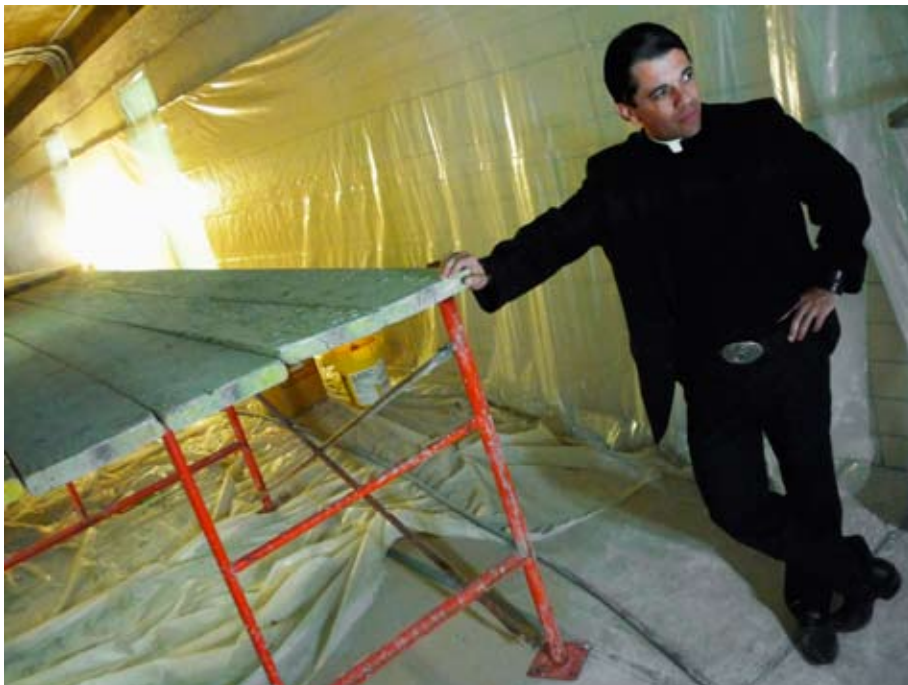
Fr. T.J. Martinez, SJ, has a dream coming to fruition: a Cristo Rey School in Houston, welcoming 100 students this fall. He and his team secured over $2 million in grants and donations to renovate an old school near the city's Hobby Airport. www.cristoreyhouston.org
