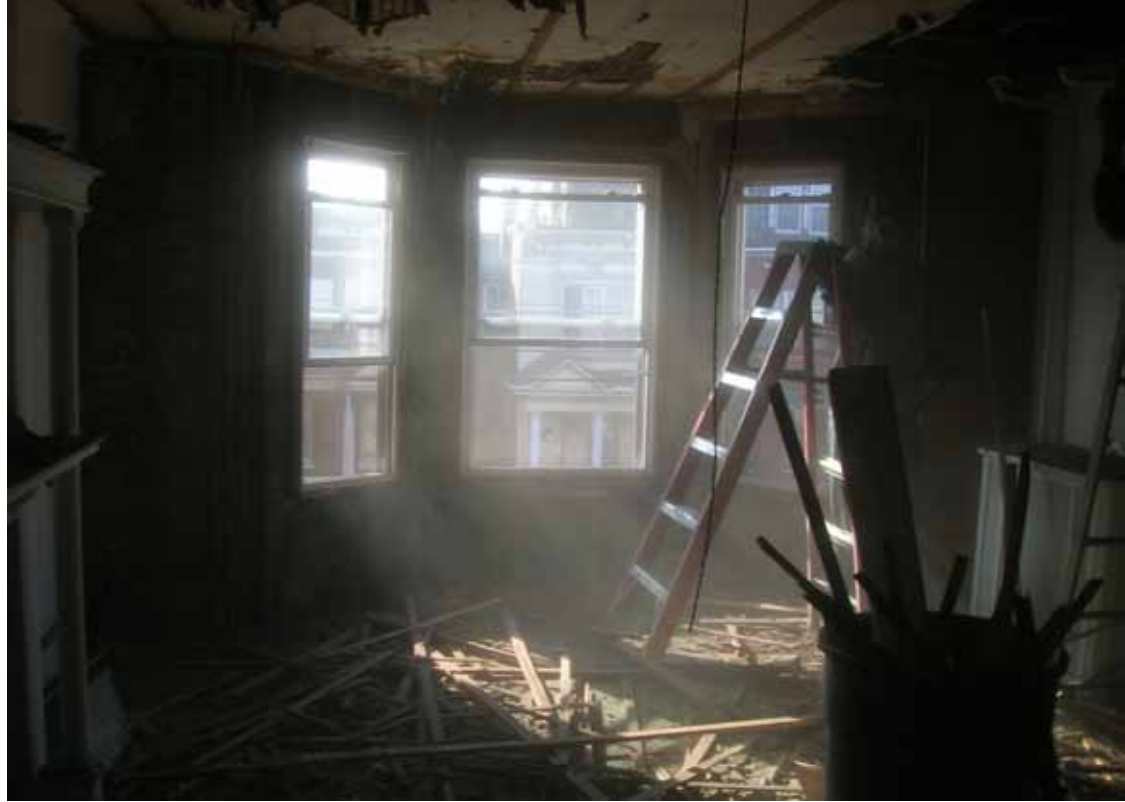
Renovation is underway at a donated building that will be housing for former Hopeworks participants who are working or going to college and need a stable living environment.
